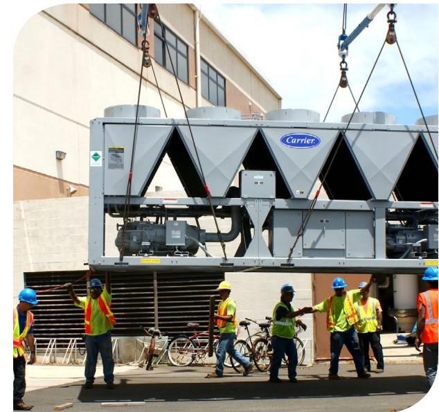
FEMP chiller being installed at Navy Facility. Photo credit: U.S. Navy photo by Thomas Obungen/Released
